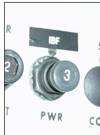
Picture 3: Circuit Breaker
